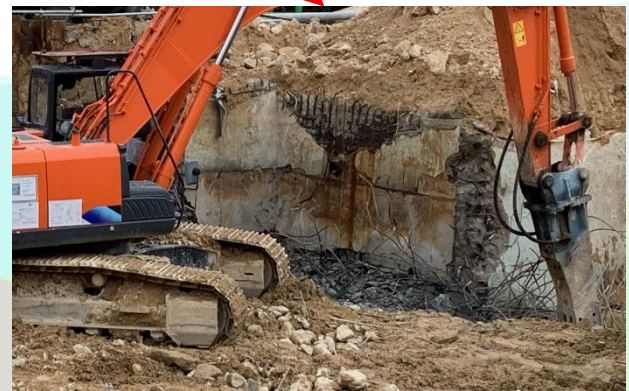
Demolition of Existing Substructure at Preliminary Treatment Facilities 基本處理設施拆卸工程
