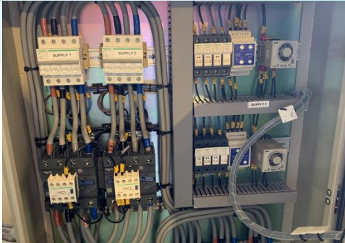
Installation of Temporary Automatic Transfer Switch System inside LV Main Switch Room 在總制房安裝臨時自動轉換開關系統
